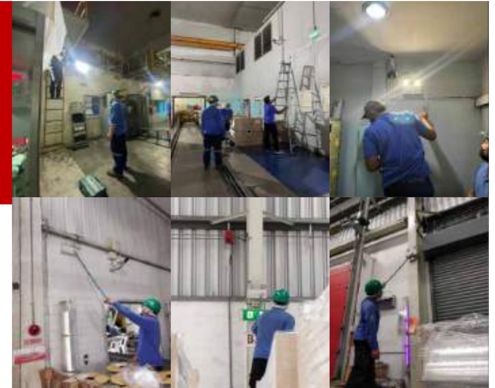
Monthly Emergency Light Inspection
