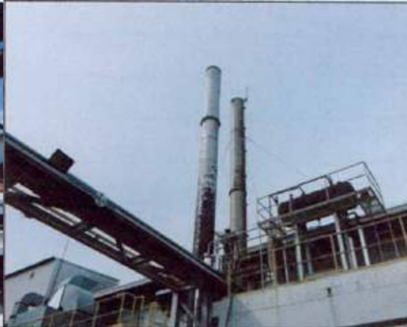
Figure 2: Air quality sampling Boiler Stack No.9 BOPET
